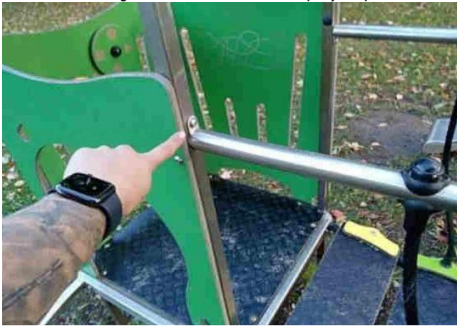
Figure 3: Loose Fittings ( Low)
