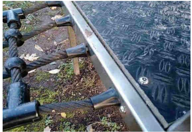
Figure 4: Loose Fittings (Low)
